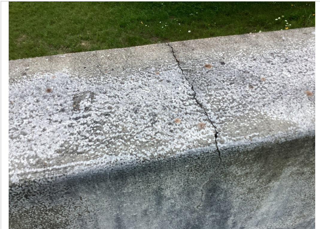
Parapet crack typical
