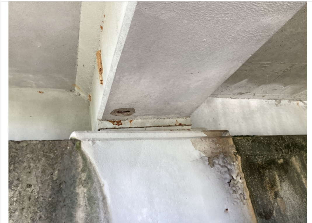
Span 1 beam B spall to steel
