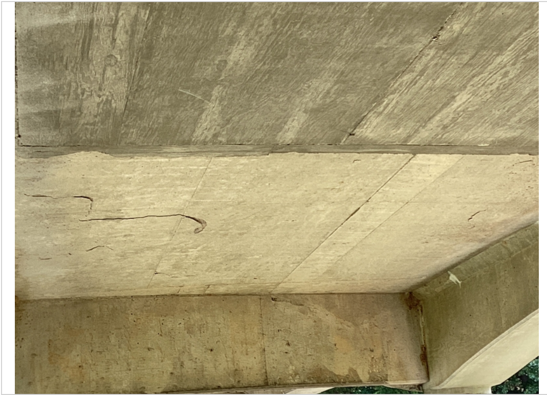
Span 1 bottom deck impending spall typical
