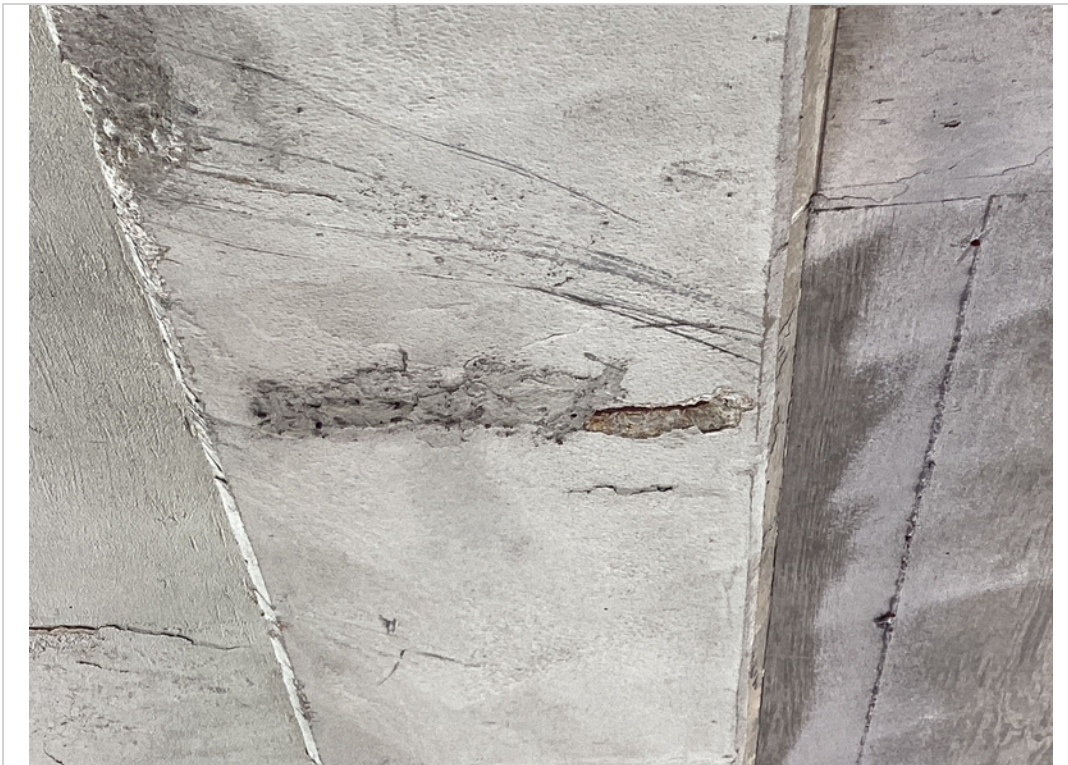
Span 1 beam A spall to steel
