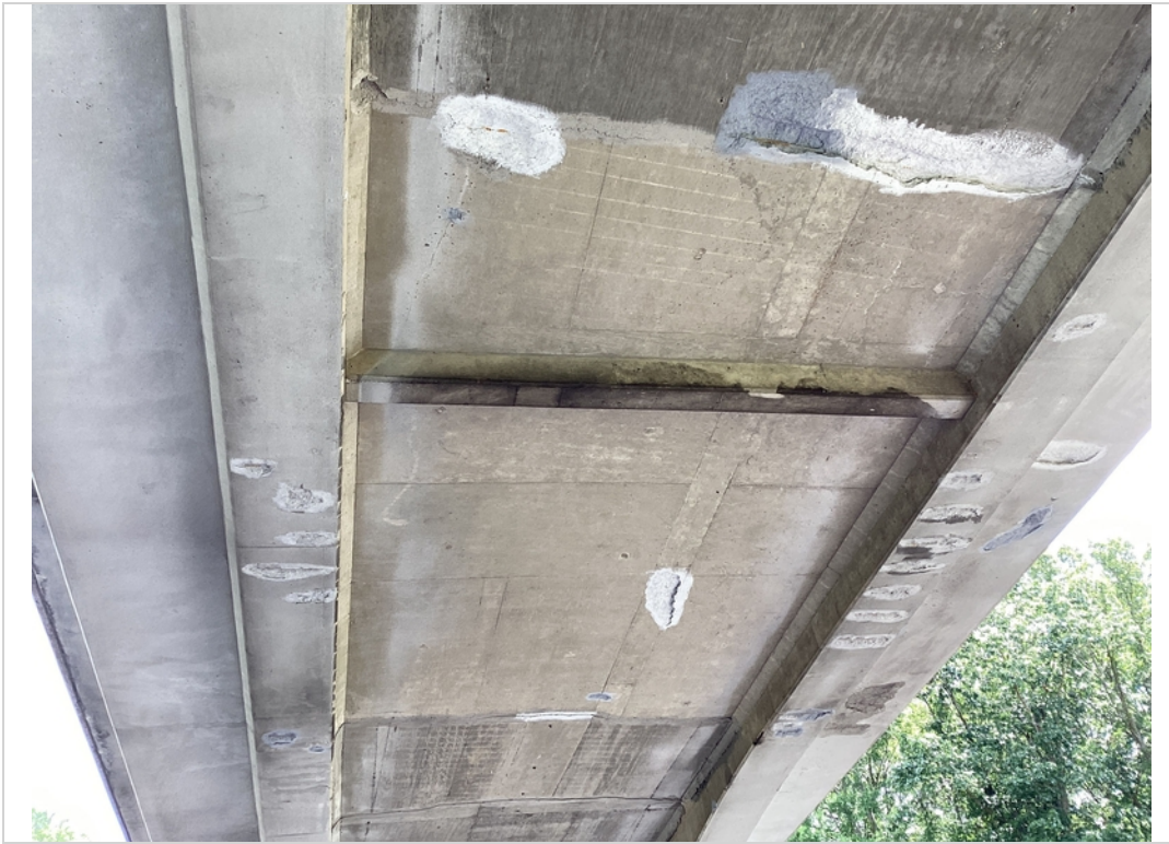
Bottom deck span 2 typical with spall to steel in deck and girders
