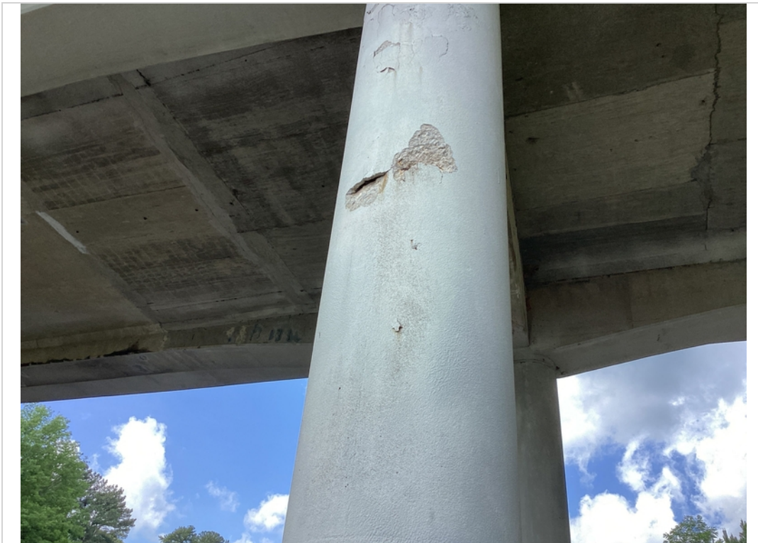
Spall steel bent 1 column b
