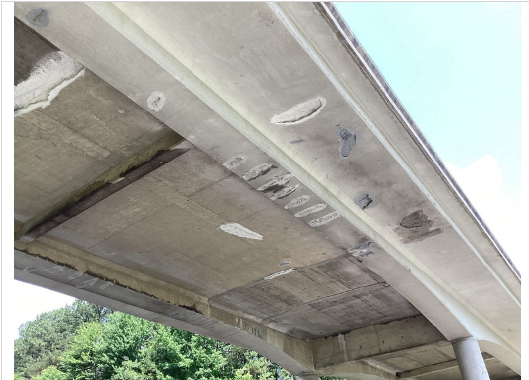
Bottom deck span 2 spall to steel
