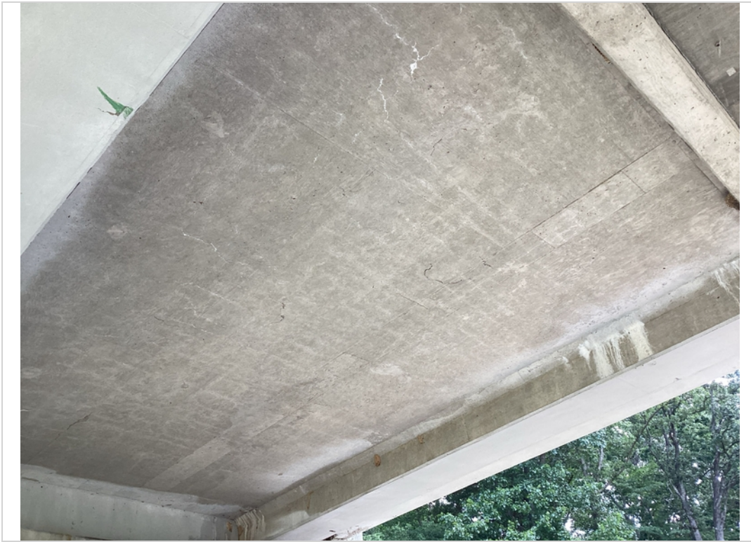
Impending spall on bottom deck of span #3
