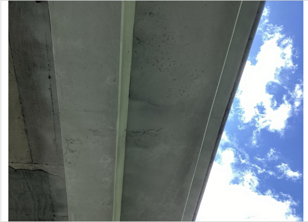
Impending spall on bottom deck of span #3
