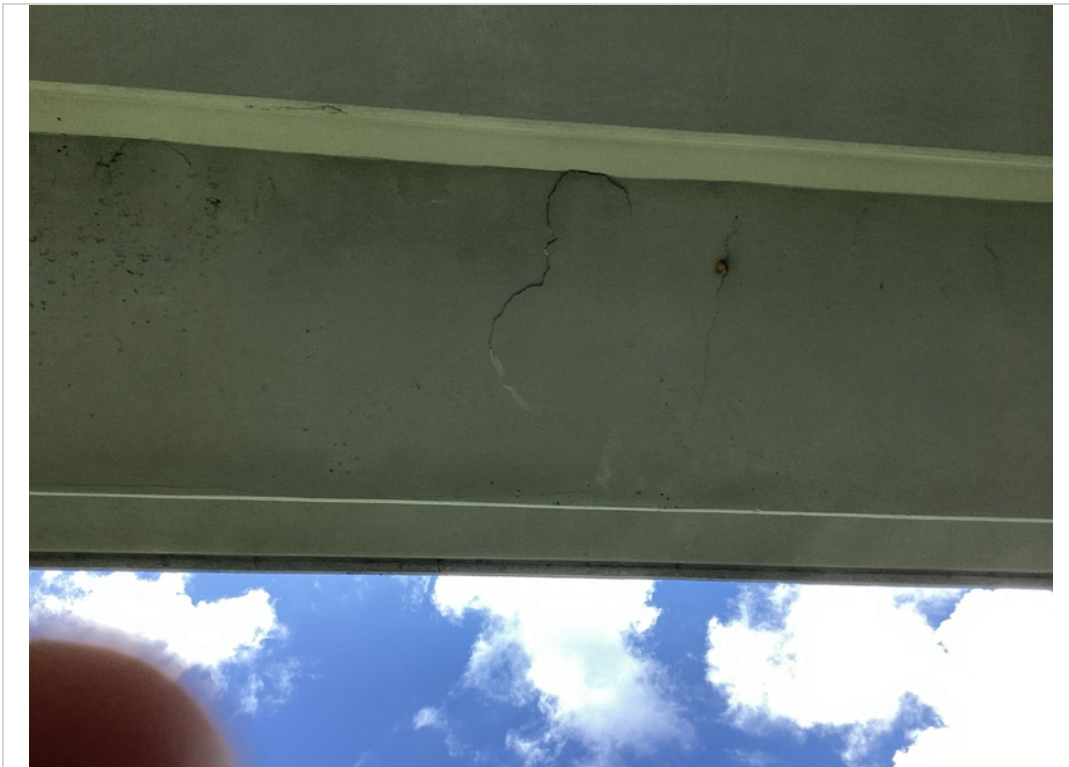
Impending spall on bottom deck of span #3
