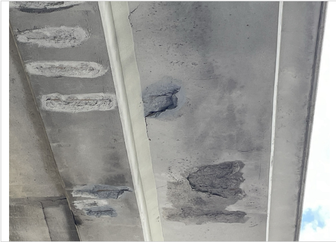
Span 2 right overhang impending spall
