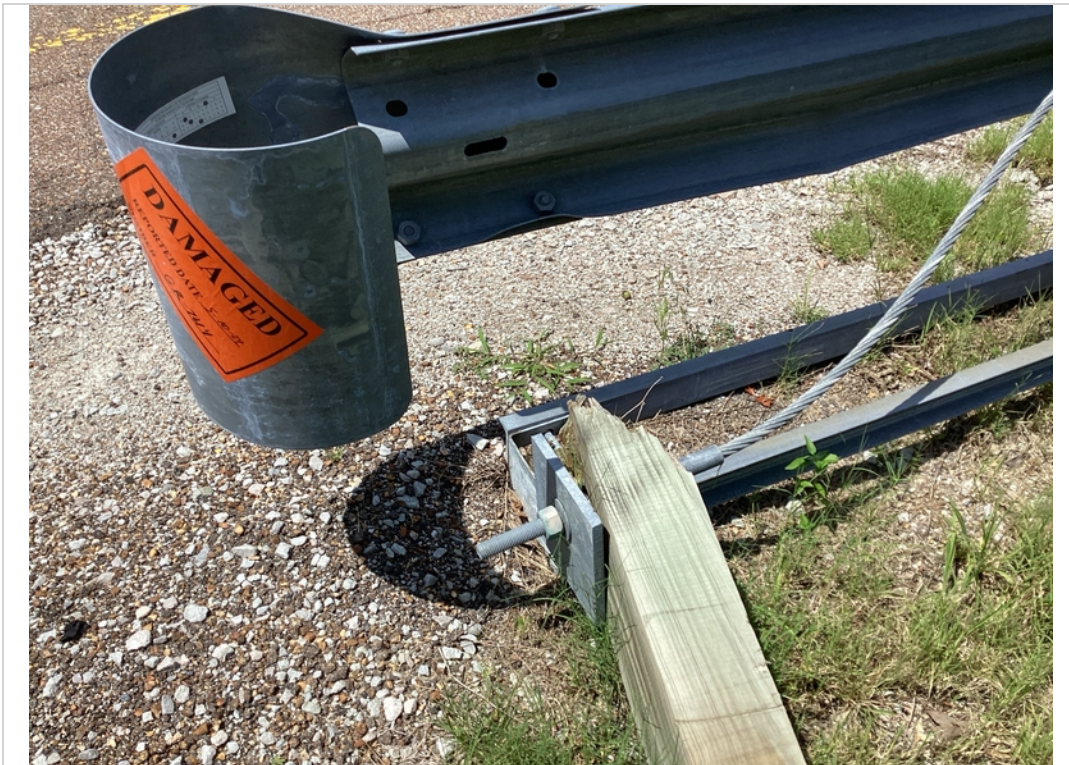
Approach 1 right terminal damage
