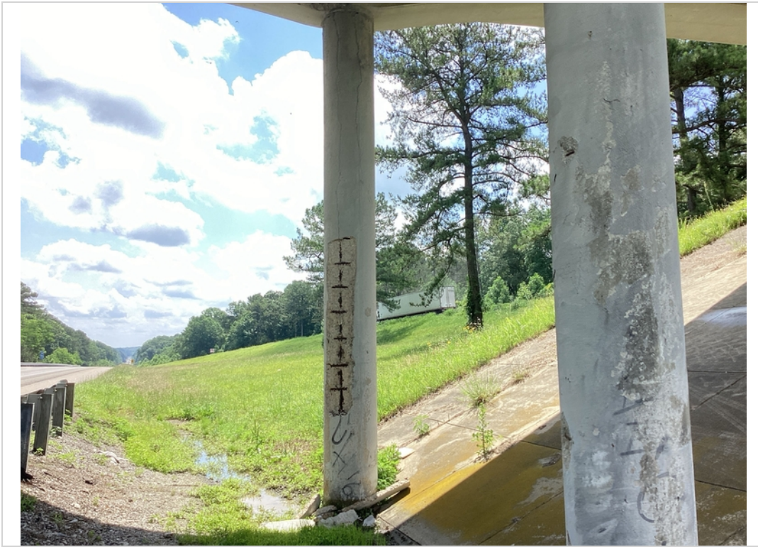
Bent #1 column B spalling
